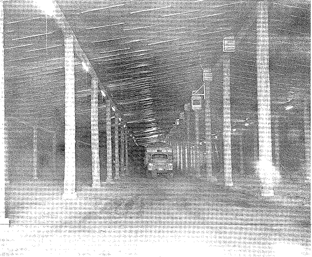
Fig. 3. Inside view of Fig. 2. Note how vapor barrier and chicken wire netting is held up by lath. Photo courtesy of U. P. Railroad.
