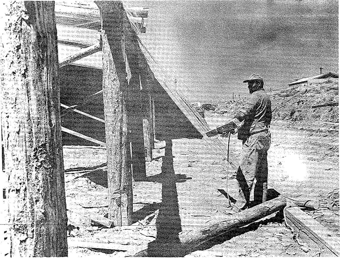
Fig. 7. Construction view of Fig. 2 showing foundation and footing detail. Courtesy of U. P. Railroad.
